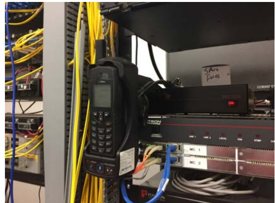
Telecom shelter servers. Published with permission from Western James Bay Telecom Network (Ontario).
