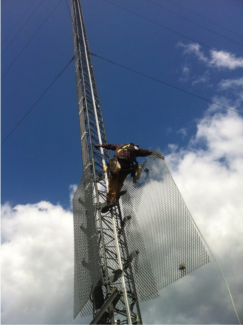
Installing components on a cell tower, Published with permission from Keewaytinook Okimakanak KNET Services (Ontario).
