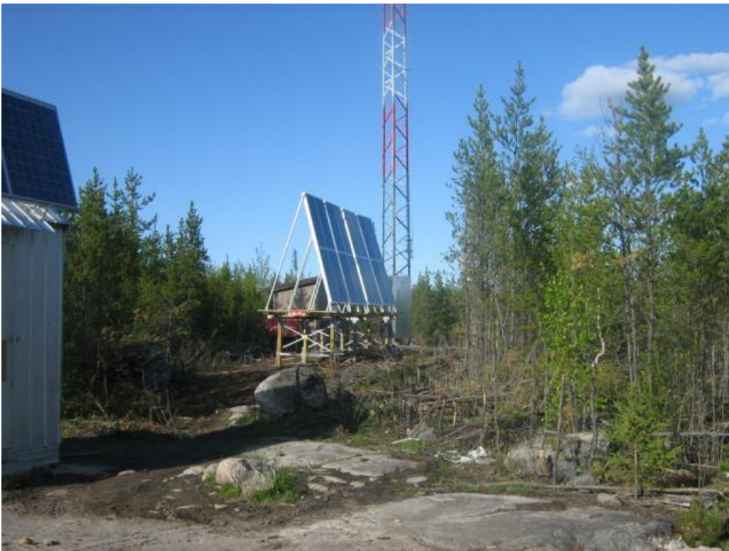
Figure 3: Photo of the solar-powered cellular tower and radio equipment erected in Summer 2008 at Koocheching First Nation, Ontario (photo from the K-Net Media archive http://media.knet.ca ).
