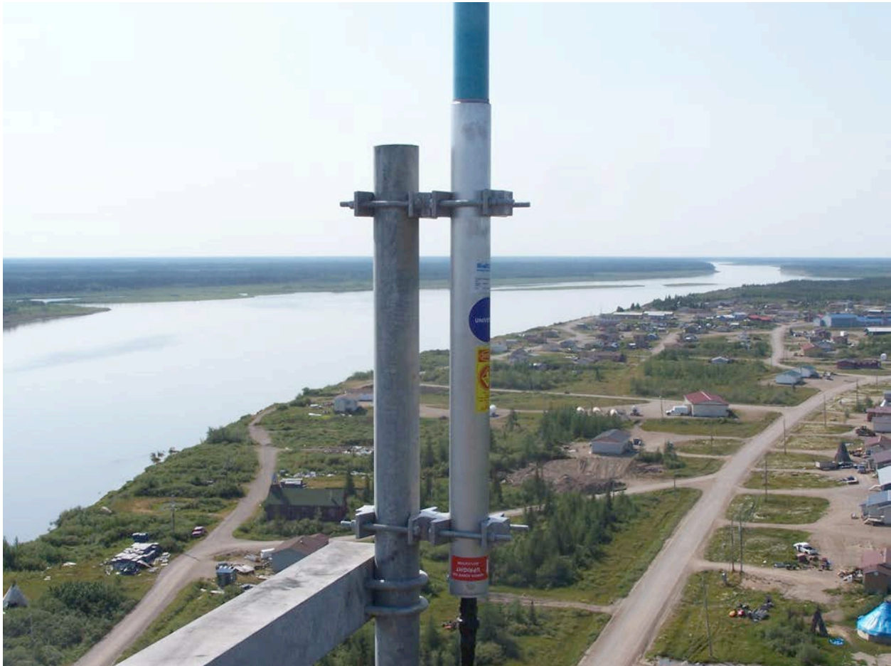
Figure 2: Installing the cell tower in Fort Severn First Nation, 2009 (photo credit KO-KNET)
